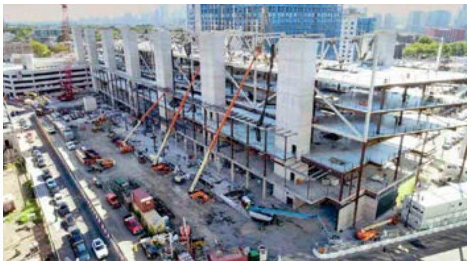
Hudson County's new Frank J. Guarini Justice Complex was constructed under a Project Labor Agreement (PLA).
