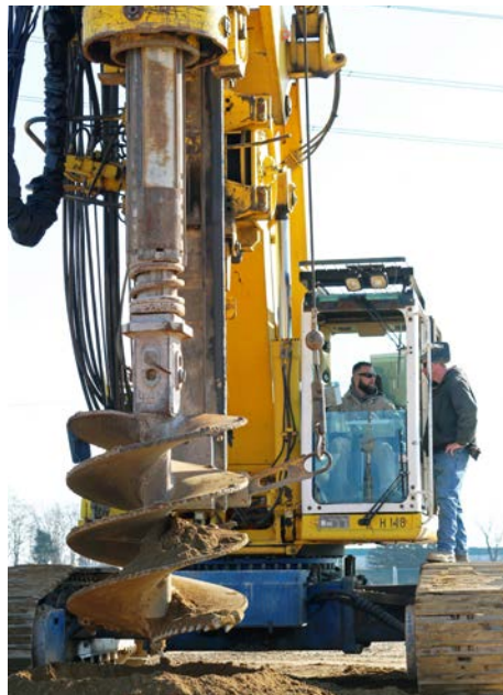
Ryan Spirito and Warren Kuhlthau take turns on the Bauer drill. This and the Casagrande drill will be offered for training during winter classes.
