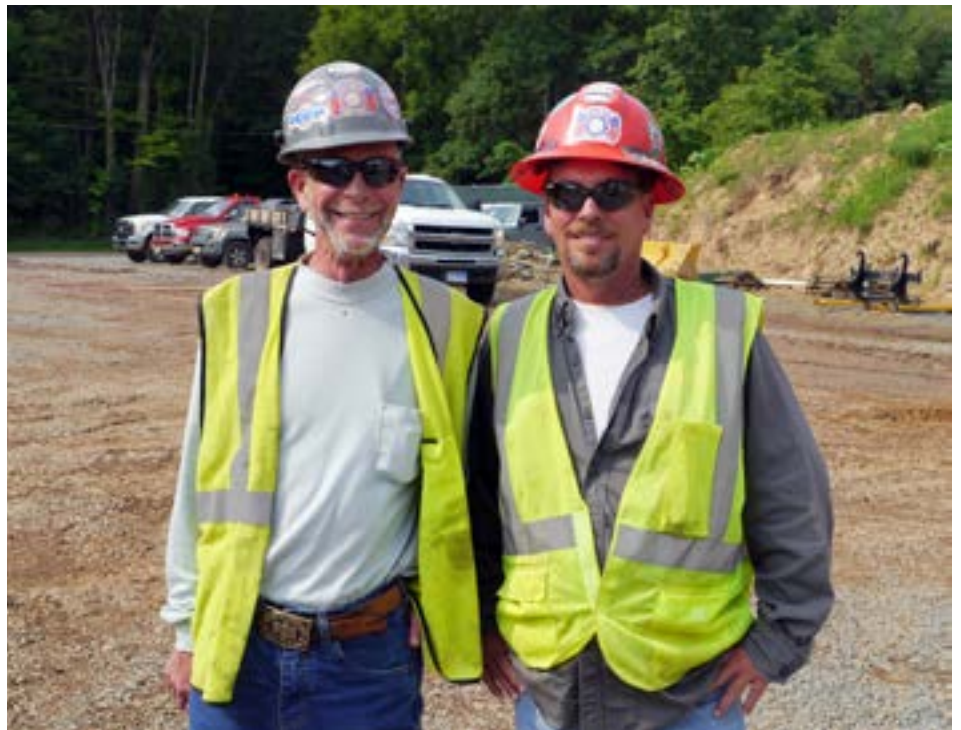
Fellow lead engineers Pat Flynn, a 39-year veteran and Joe Eichele, at 31 years reviewing the Cherry Valley Road worksite.
