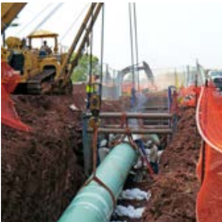
This photo shows how this pipeline crosses through some neighborhoods.
