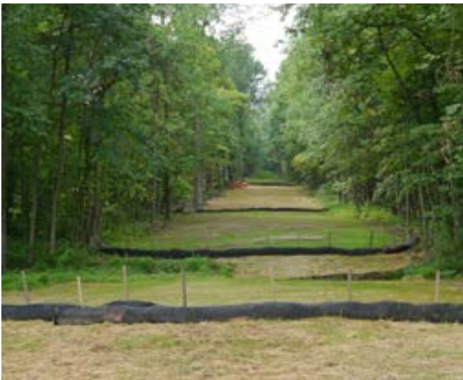
Once work is done, gravel and matts are removed, the area is graded, seeded and restored to its prior condition.
