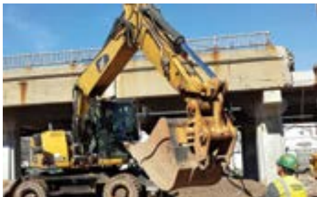
Demolition crews cut sections of the bridge to make room for the Bauer drill rig.
