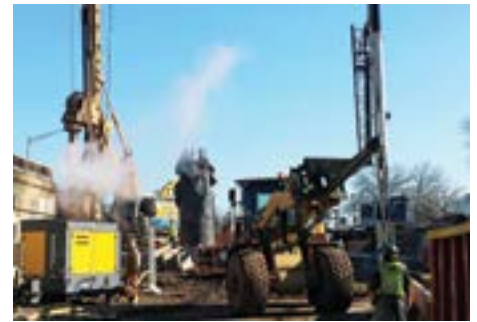
The Bauer drill rig works on footings for the precast concrete sections that will be used to support the approach roadway.
