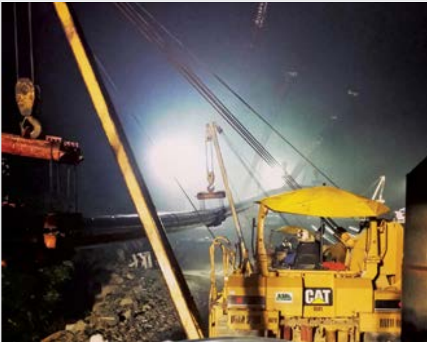
Directional drilling throughout the night crosses 5,200 feet of the Wannaque reservation before the new pipeline is pulled back.
