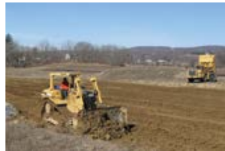
Bill Davis handles the bulldozer, grading the area for the future road and parking lot.
