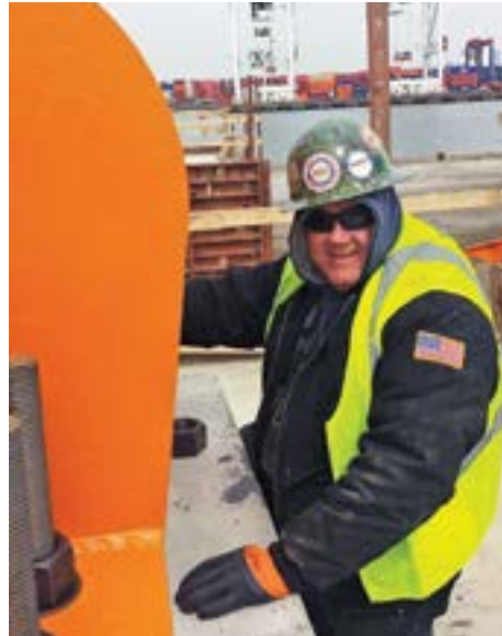
Glynn Dubil at work on the triple waterfall winch for the stiff-leg derrick.
