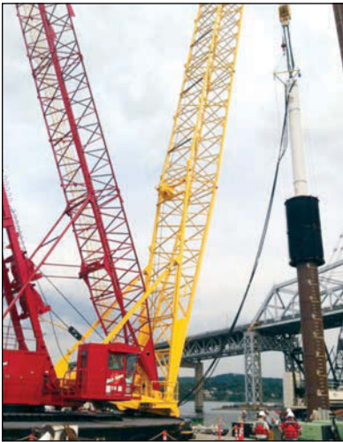
Local 825 operator Pete Cerniglia drives the first pile for the future Tappan Zee Bridge.
