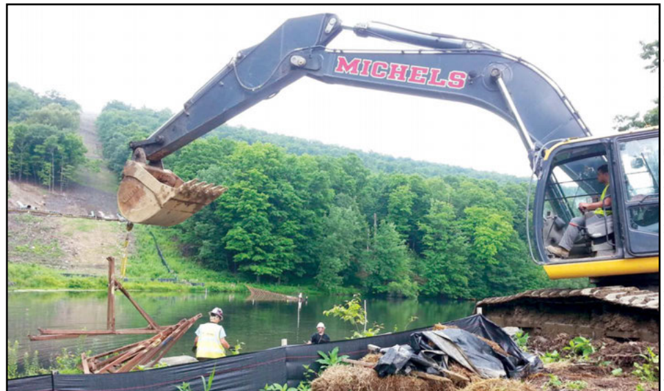
Crews construct a Portadam to separate the lake and create a dry path through wetlands of McCormack Lake, preparing the bed to lay pipe. The Portadam above-ground water storage system allows work to progress while complying with stringent state and federal environmental regulations.
