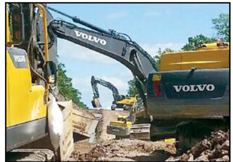
Work progresses with care being taken at every turn to protect the environment.
