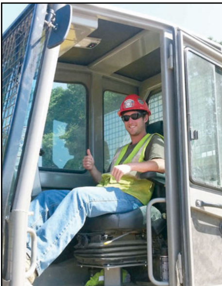
Dan Richardson, Local 825 apprentice, serves as an oiler on a tie-in crew that joins sections of pipe together.
