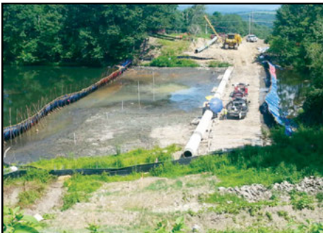
Preparing the way for Portadam installation to bring in sections of pipe across wetlands.
