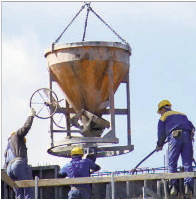
Heavy lifting is not always done by heavy equipment. Knowing the right techniques helps keep us all safe.
